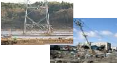
Damage to transmission lines/tower Caused the loss of offsite power
